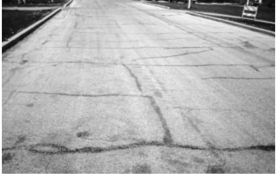
▶ Large blocks, approximately 10' across.
