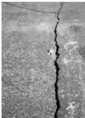
▲ Open crack – 1/2" or more in width.
