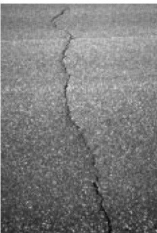
▲ Tight cracks less than 1/4" in width.
