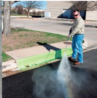
Street Curb Inlet Cover
