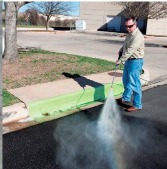
Street Curb Inlet Cover
